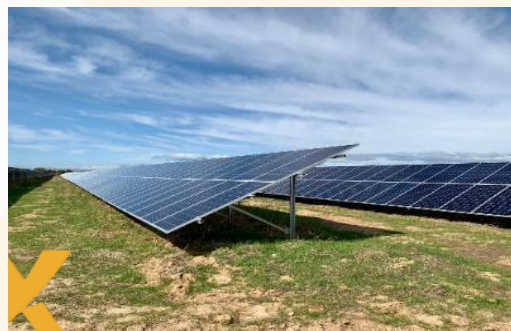
PV Cañamares (Guadalajara) 5 MWp
